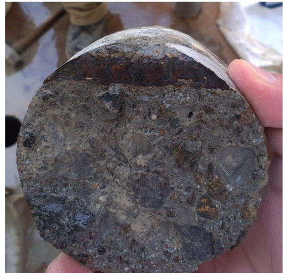
Fig. 6 Top 8mm reinforcement observed in the concrete core.
